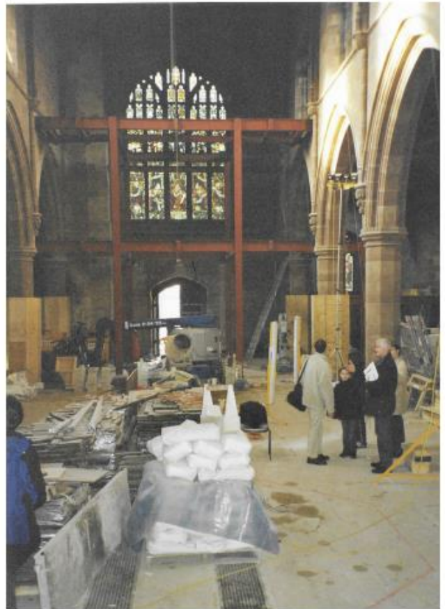
The building works underway: the view to the main entrance and west window, with the massive steel frame now in place to support the Welcome Area, the upstairs room and the choir vestry.
